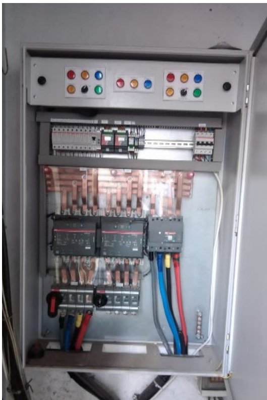
Main Distribution Board outside the facility
