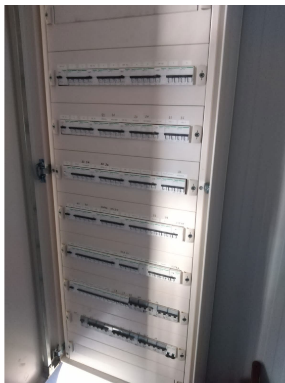
Distribution Board in the technical room
